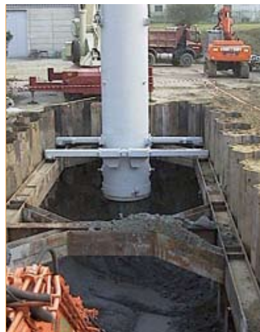
In 2008, the call for tender for the extraction of the remaining 14 pits was completed.
