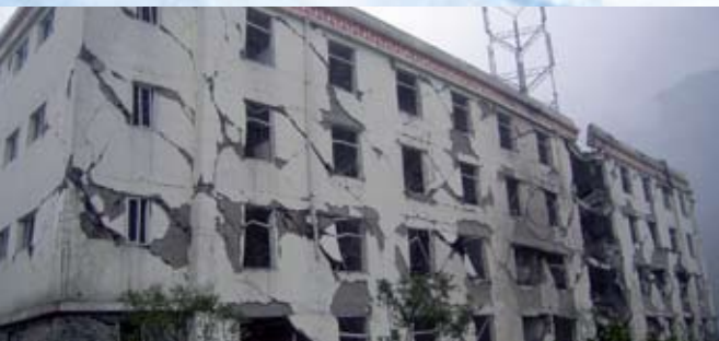
Yingxiu town of Wenchuan County: soft storey collapse of a Xu-ankou middle school five-storey building.
